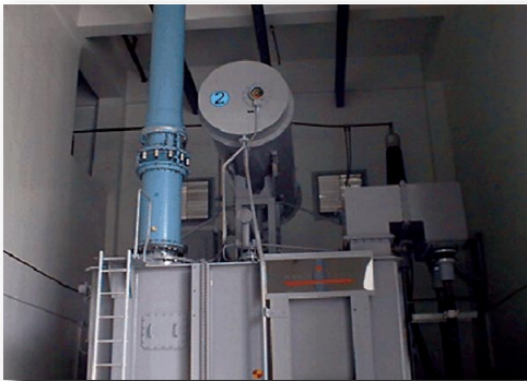
▲ Problem detected - bushing defects
